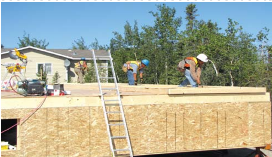
The Tli Cho Construction crew of Floyd Flunkie, Frank Black and Shane Football are hard at work preparing to stand up an exterior wall on an NWTHC 3-bedroom detached unit currently under construction in Behchokò. (Photo by Curtis Coleman)
