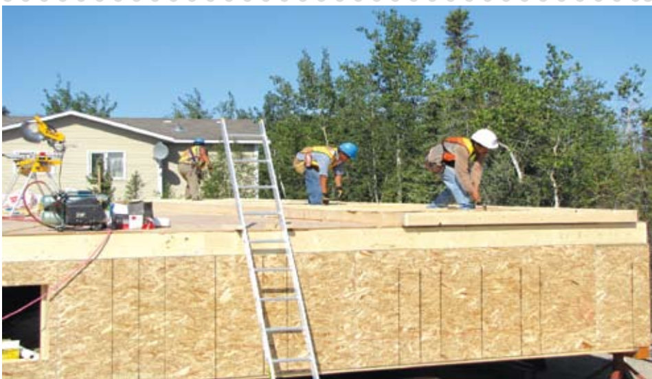
The Tli Cho Construction crew of Floyd Flunkie, Frank Black and Shane Football are hard at work preparing to stand up an exterior wall on an NWTCH 3-bedroom detached unit currently under construction in Behchokò. (Photo by Curtis Coleman)
